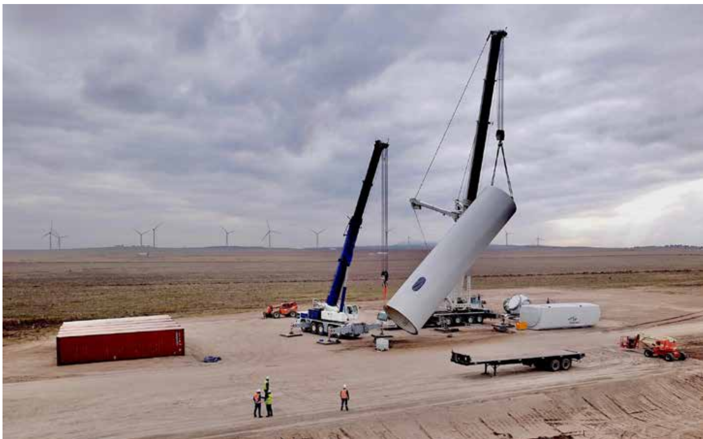
Erecting locally manufactured wind turbines at PE Los Olivos (Argentina, late 2019). Photo courtesy of Central Puerto Renovables S.A.
